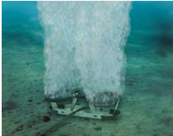
Figure A.6 - Submerged Tailrace Diffusers
